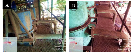
Gambar 4. Kondisi unit hydrocyclone
