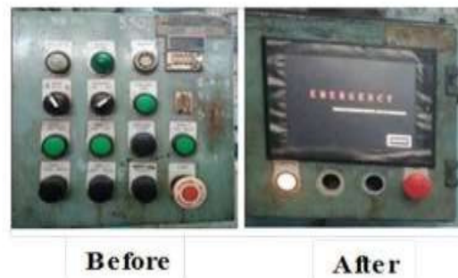
Figure 13. Machine control panel modified
